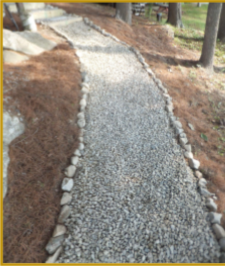
Infiltration Path - a trench filled with crushed stone that traps stormwater. Can replace dirt paths susceptible to runoff.
