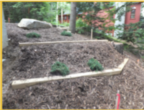
Water Bars - 6"x 6" lumber is installed on a slope with crushed stone on the uphill side to trap and divert stormwater. Water bars are left slightly raised to slow water down and can be used as seen above, or placed in a pathway in shorter lengths to function as steps.
