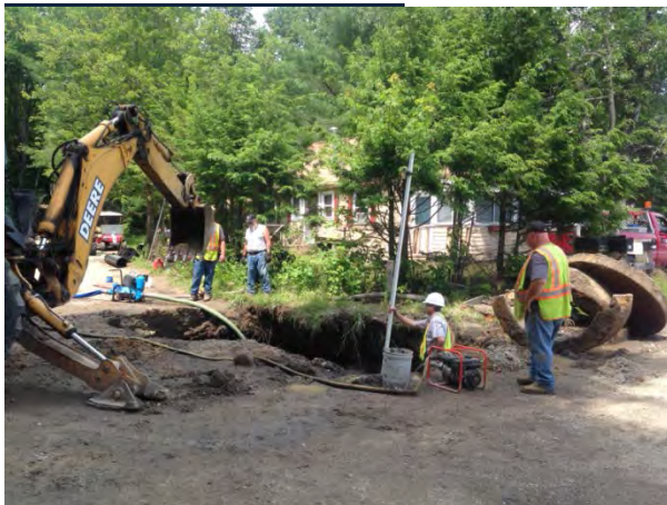
Figure 8: Jamie Houle, UNHSC and the Wakefield Highway Dept installing BMPs on Bonnyman Road.
